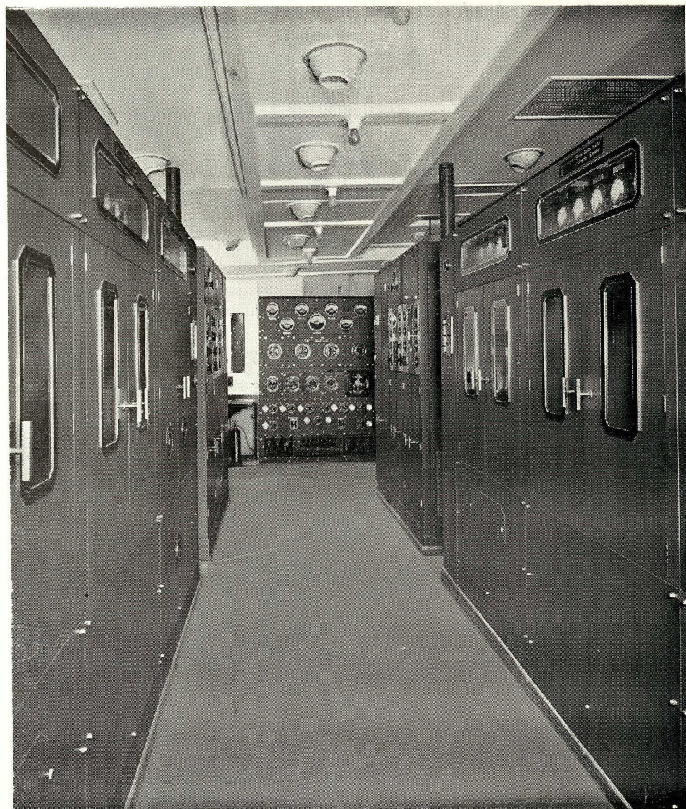
This view in the Radio Transmitter Room on board the "QUEEN MARY" gives some idea of the size of the great transmitters which are remotely controlled from the Radio Control Room 400 feet away.
